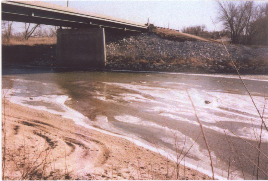
Figure 1-1 Many bridges are constructed with a pier in close proximity to an abutment.
