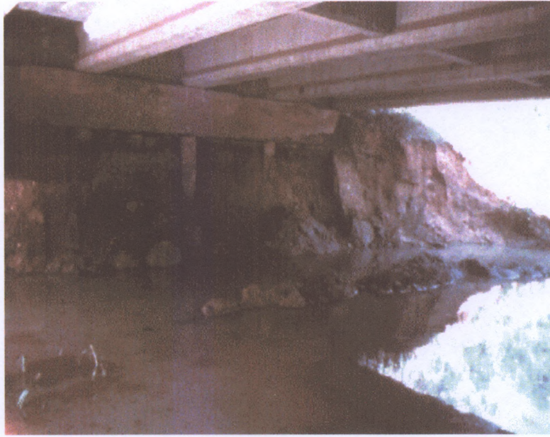
Figure 2-7 Hydraulic erosion of earth-fill embankment
